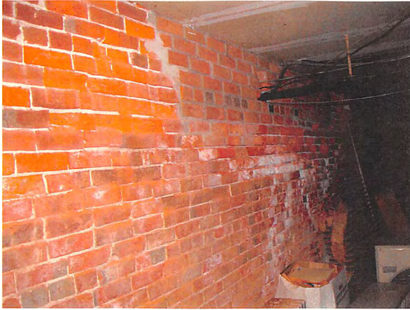
Interior brick wall requiring re-pointing
