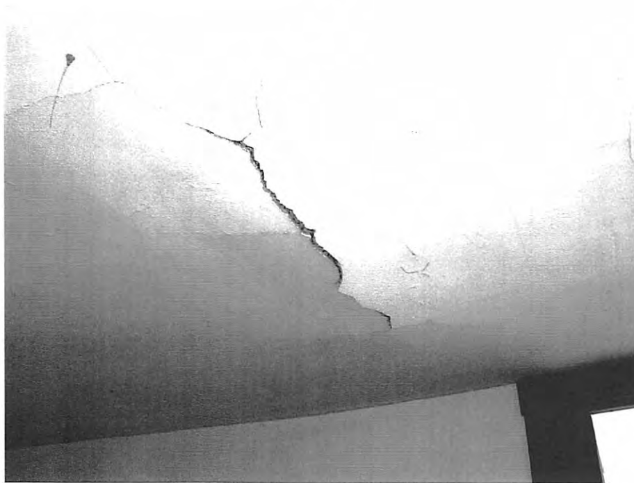
SECOND FLOOR LOBBY CEILING Cracked Plaster
