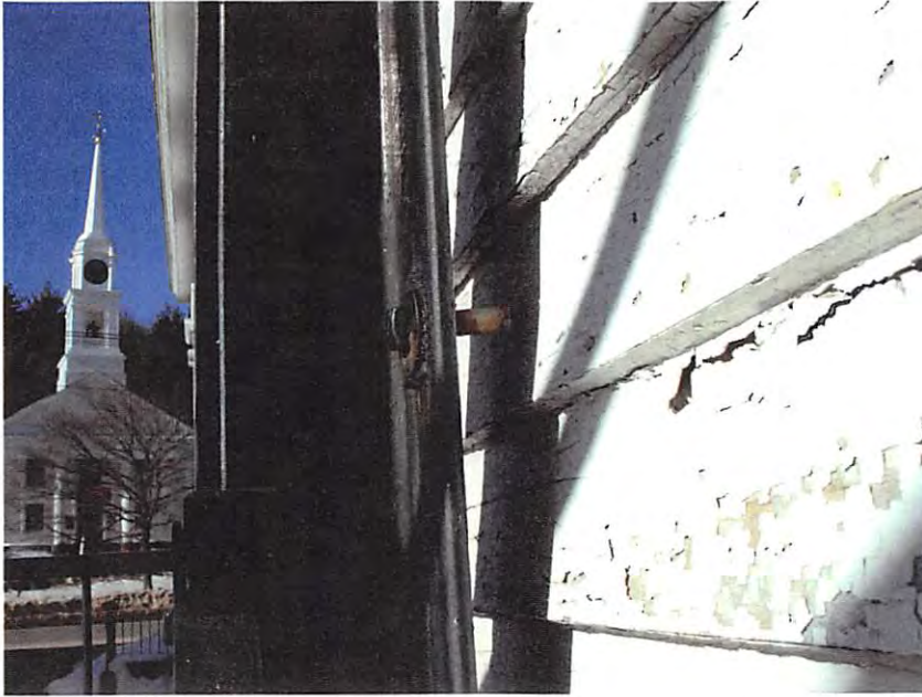
Inadequate anchorage of Fire Escape
