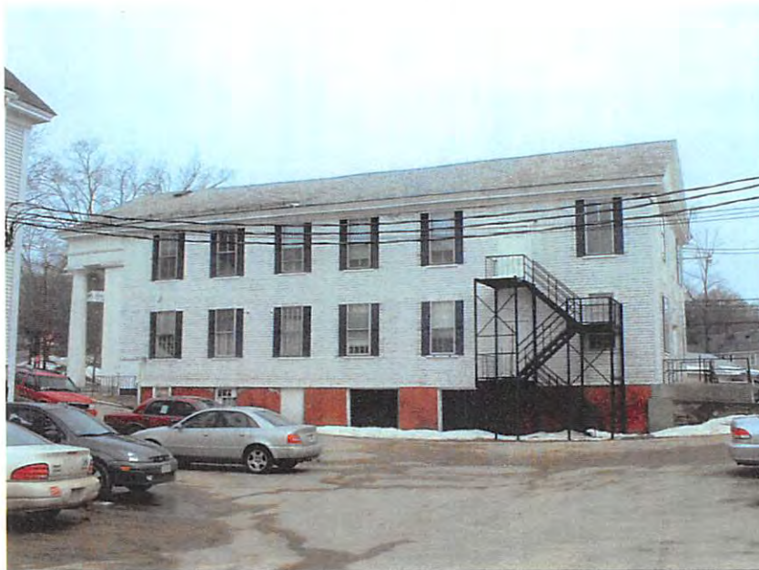
Right Side Building Elevation – Hump in Roof Ridge
