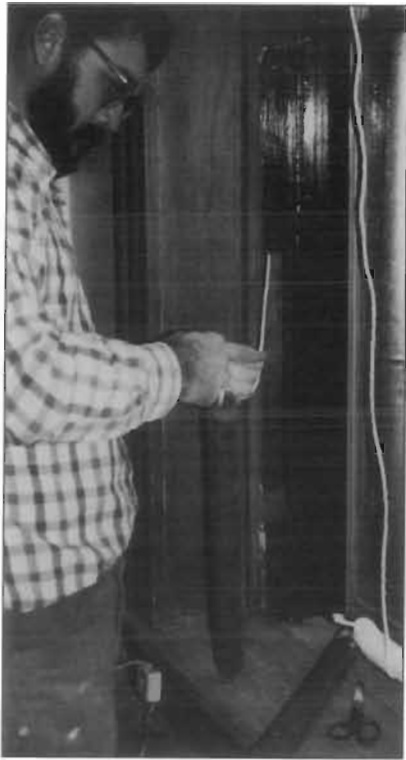
Maintaining a historic window may include work as basic as replacing a sash cord.
