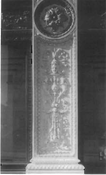
The decorative cast-iron storefront column was sandblasted in order to remove flaking paint and rust prior to repainting. Unlike soft metals such as copper and tin, which are damaged by abrasive cleaning, sandblasting is an appropriate method for cleaning cast iron, a very hard metal.
