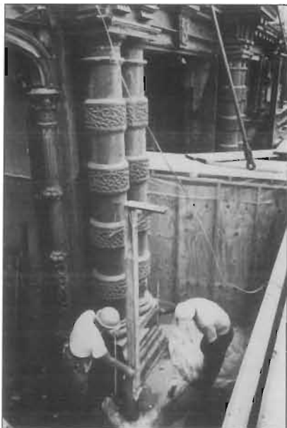
The cast-iron columns of this theater are being repaired during rehabilitation. Some of the cast iron elements such as the smaller, non-structural columns missing from the bay on the right will be replaced with a lightweight substitute material such as cast aluminum, an acceptable alternative according to the Standards.
