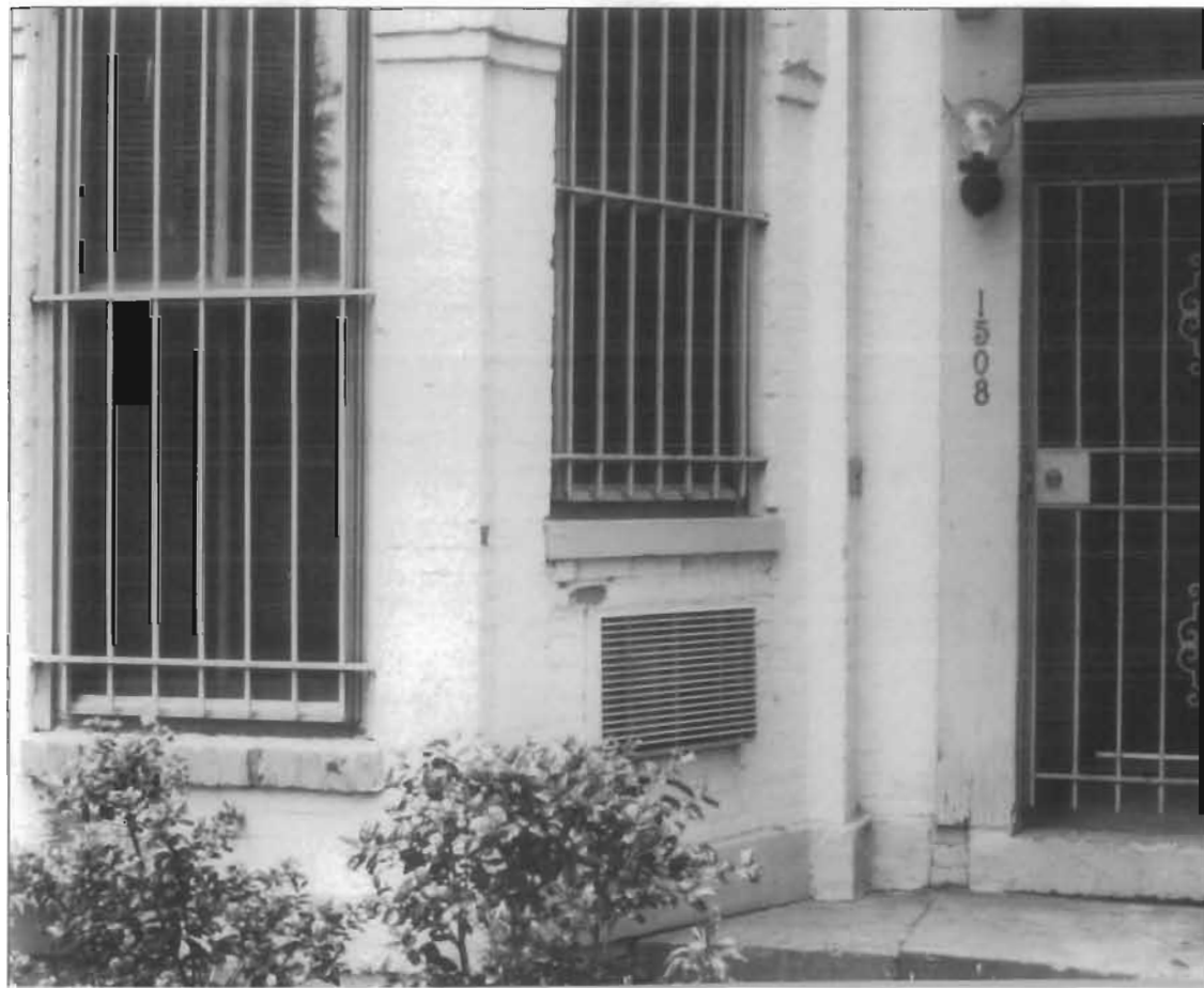
The historic window on a primary facade has been shortened and the area below it filled in with brick in order to install a through-the-wall air conditioning unit. In addition to changing the window size and destroying the sill, the unit itself is visually obtrusive.
