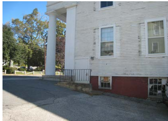
Cracked and stained concrete entry platform at the northwest corner. Painted masonry foundation with failed mortar joints and peeling paint.
