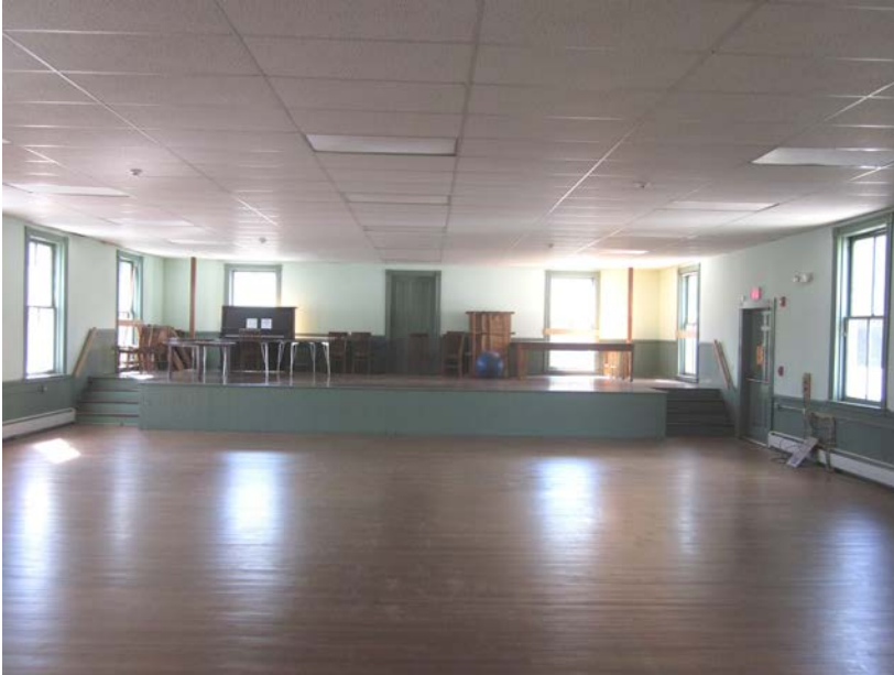
Second floor: Stage at south end of the Assembly Room. The rear window was blocked in when the stage was installed. The egress door at right was converted from a window when the fire escape was installed.
