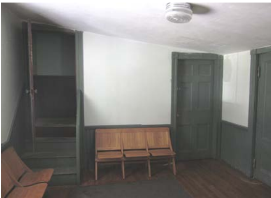
Stairs to the assembly room balcony, which has been covered by the drop ceiling. Wood doors, trim and wainscot are among the remaining original Greek Revival details at the building interior.
