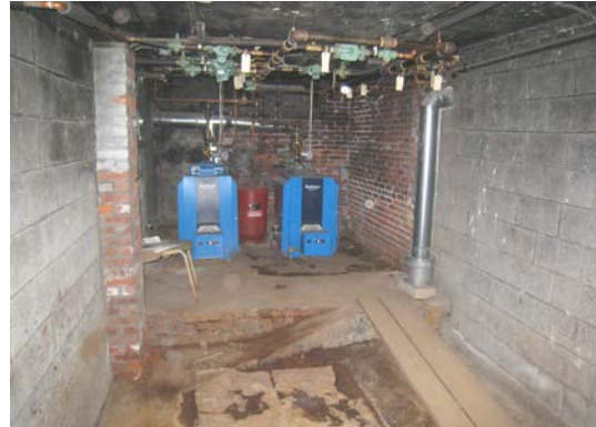
New boilers installed in the basement. Areas of moisture seen on the floor.
