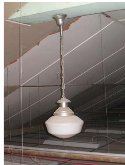
Pendant lamp obscured by drop ceiling.
