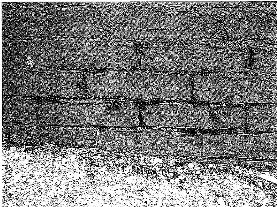
FIRST FLOOR WINDOW SOUTH ELEVATION • Moss Growing in Mortar Joints
