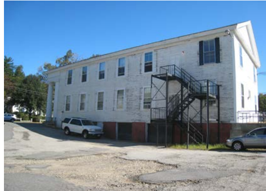
Poor paint conditions at the west elevation.
