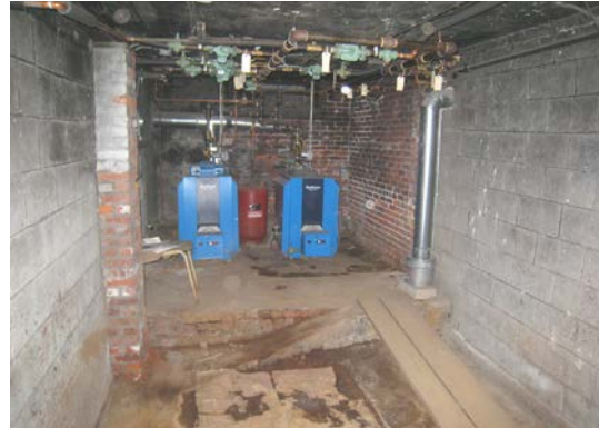
New boilers installed in the basement. Areas of moisture seen on the floor.
