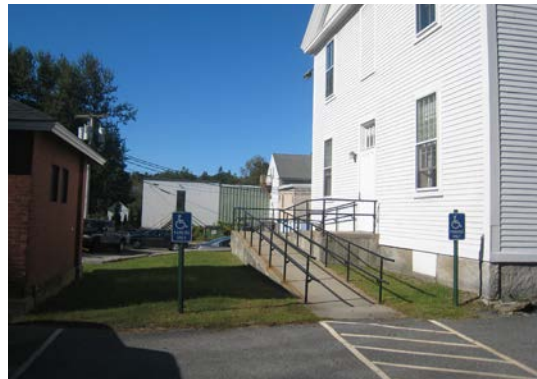
The concrete handicap ramp is in poor condition.
