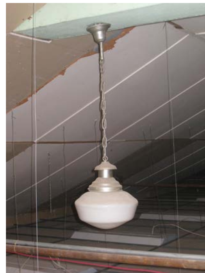
Pendant lamp obscured by drop ceiling.
