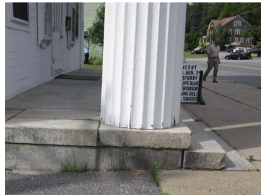
Shifted, separated granite steps at the south elevation. Paint failure at the column base.
