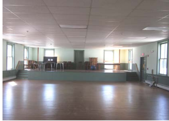
Dropped ceiling detracts from the aesthetics of the assembly room.
