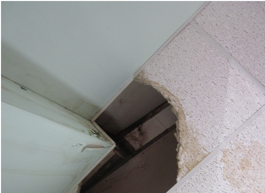
Water damage to acoustic tile ceiling.
