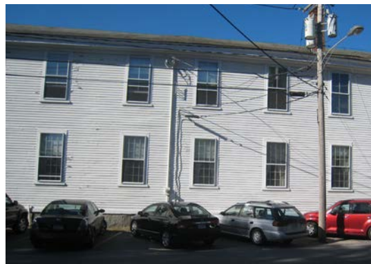
Peeling paint on wood siding around windows at both floor levels.
